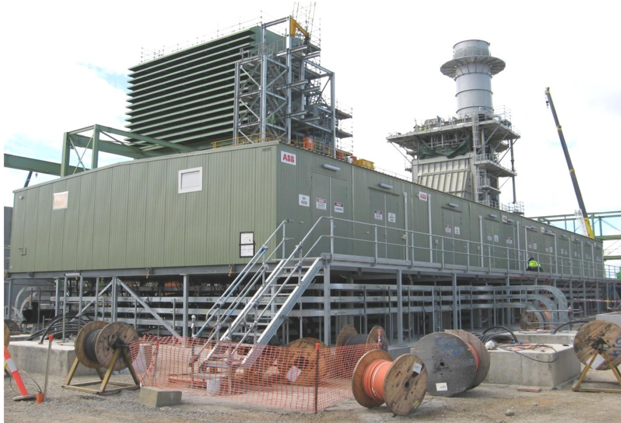
12 x Complexed E-Houses for Coal Fired Power Station
